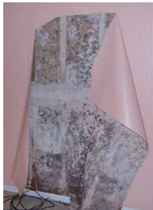
Mould hiding behind wallpaper
